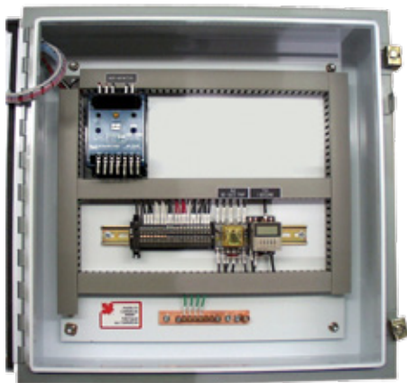
For information about the NGRM-ENC NGR Monitor Control Panel, see Accessories.
