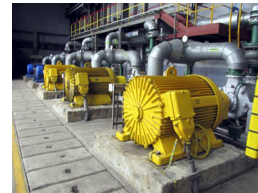
(c) Industrial water pumping station
