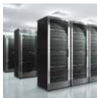
Data Center & Cloud Infrastructure
