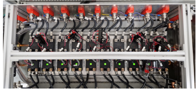
FIGURE 3. Chiller Plate with Mounted SSRs
