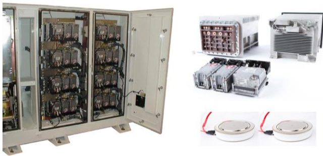
Fig. 8 Traction Inverter cabinet after refurbishment
