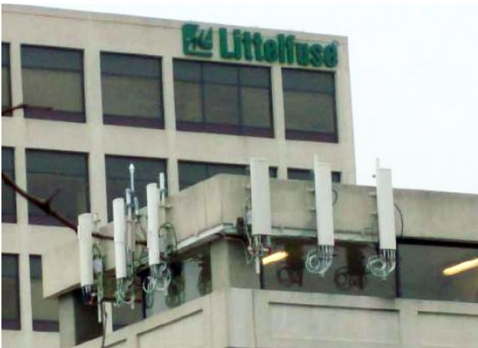
Figure 5: Zero-footprint BTS installed on the top floor of a parking garage.
