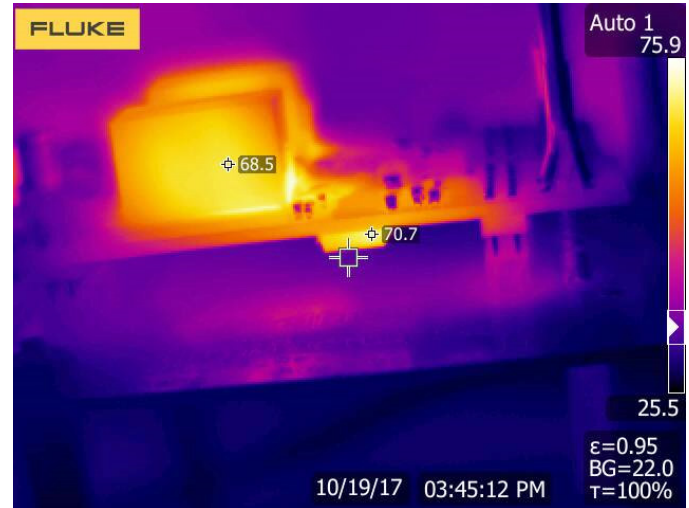
Figure 19: Thermal image of the LSICRD-GD-ISO5852 with ISO5852S and 2 Ohm gate resistance operating at 200 kHz
